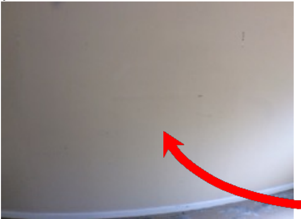
Walls/Paint - Marks on walls.
