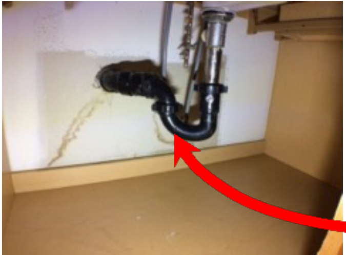
Bathroom 2 Cabinet Under Sink Discolored rear of cabinet.
