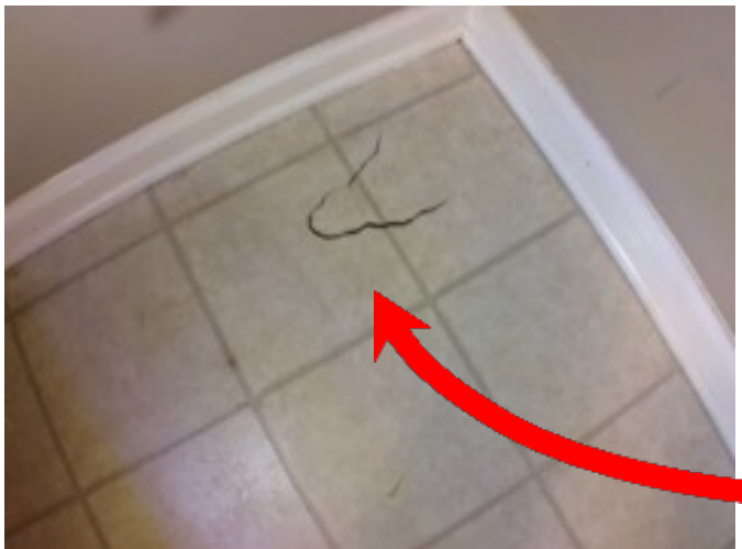
Utility Room Flooring Tear in floor.
