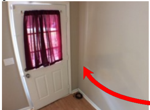
Door Stops - Missing- no wall damage noted.
