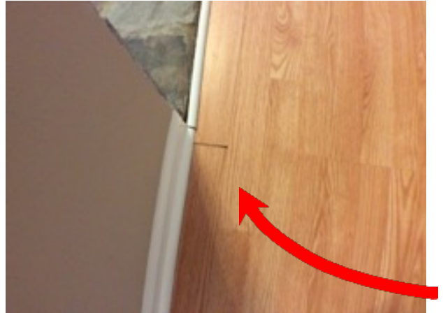
Flooring - Gap in flooring
