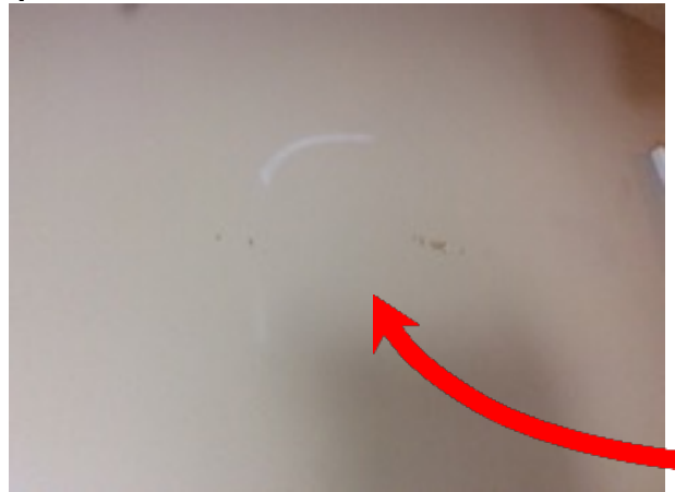
Walls/Paint - Marks on walls.
