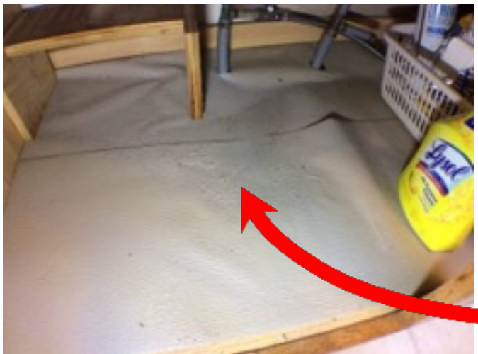
Kitchen Cabinet Under Sink There is moisture present.
