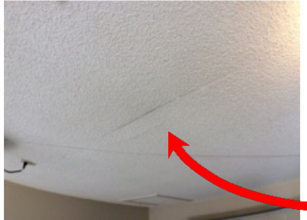
Ceiling - Cracks in ceiling.
