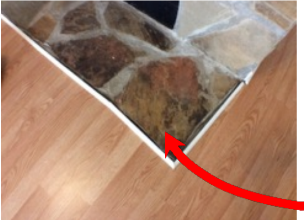
Flooring - Trim on floor not even.
