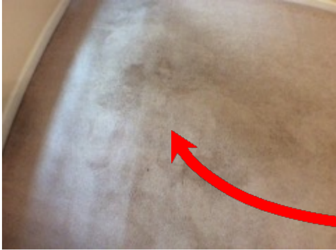
Bedroom 3 Flooring Stains in Flooring.
