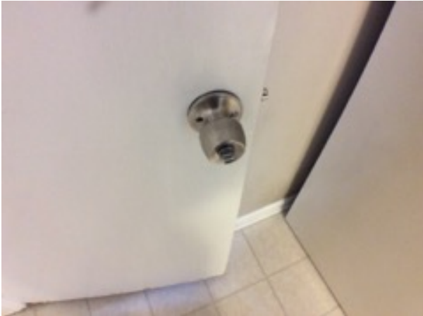
Passage Door Keyless Locks/Deadbolt - No deadbolt installed.
