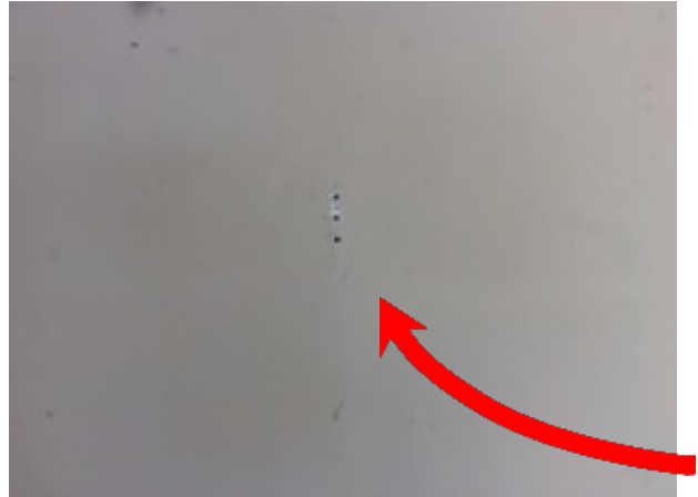
Walls/Paint - Holes in wall.
