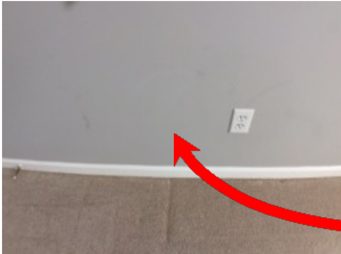
Bedroom 2 Walls/Paint Marks on wall.
