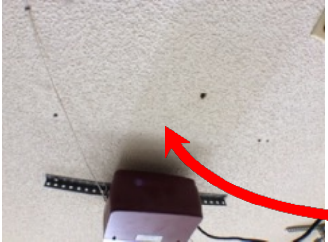
Garage Ceiling Holes in ceiling.
