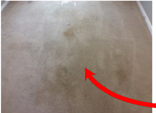
Flooring - Stains in Flooring.
