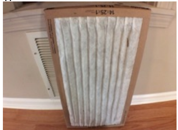
AC Filter - FILTER CONDITION: Filter very recently replaced. Little or no dust observed.
