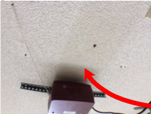
Ceiling - Holes in ceiling.
