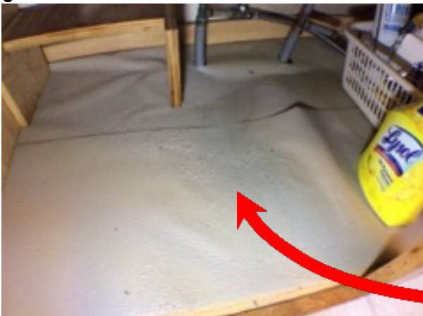
Cabinet Under Sink - There is moisture present.
