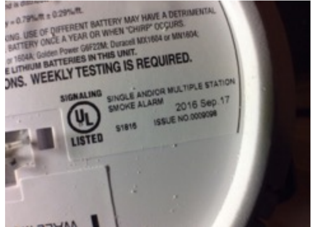
Smoke Alarm (DATE)
