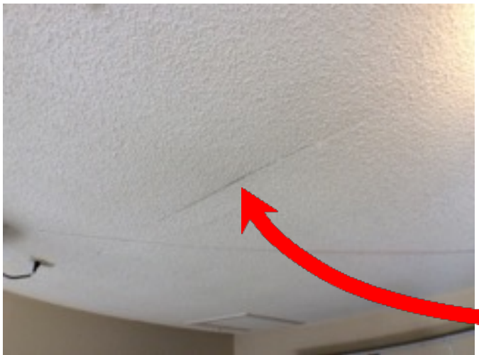
Garage Ceiling Cracks in ceiling.
