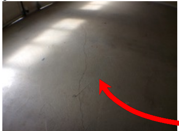
Flooring - Crack in flooring.
