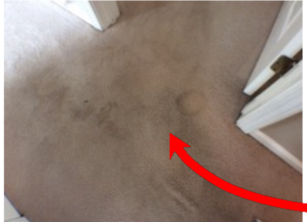
Flooring - Stains in Flooring.
