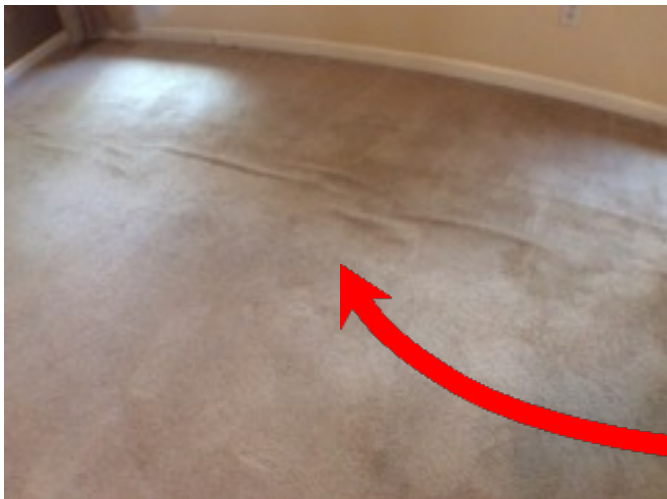
Bedroom 3 Flooring Carpet loose.
