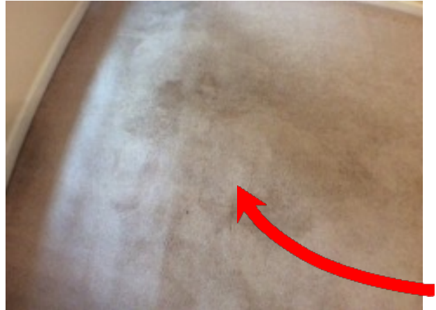
Flooring - Stains in Flooring.
