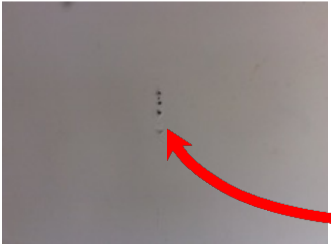
Garage Walls/Paint Holes in wall.
