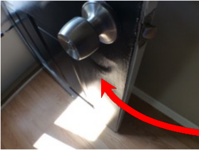
Entry Front Door Exterior Dent in door.
