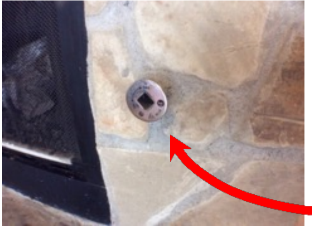
Fireplace - Fireplace key does not operate gas lever.
