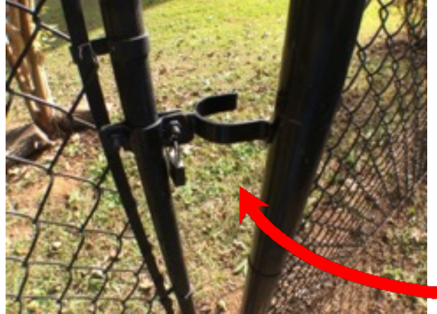
Rear Gate - Does not lock fence properly.
