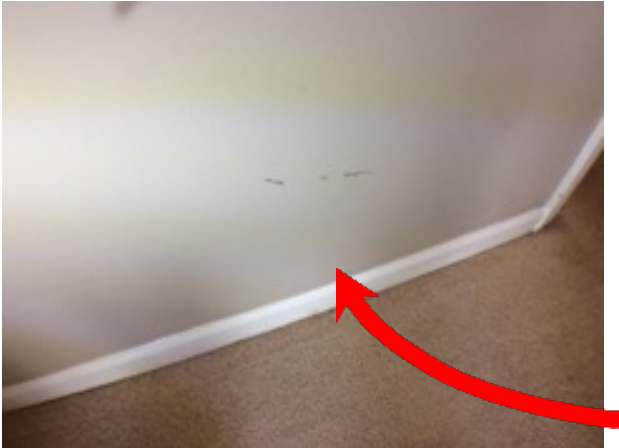
Walls/Paint - Marks on wall.
