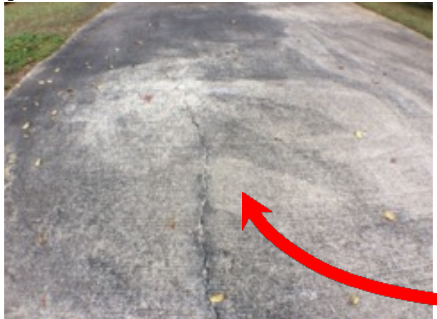
Driveway - Spider cracks in driveway.
