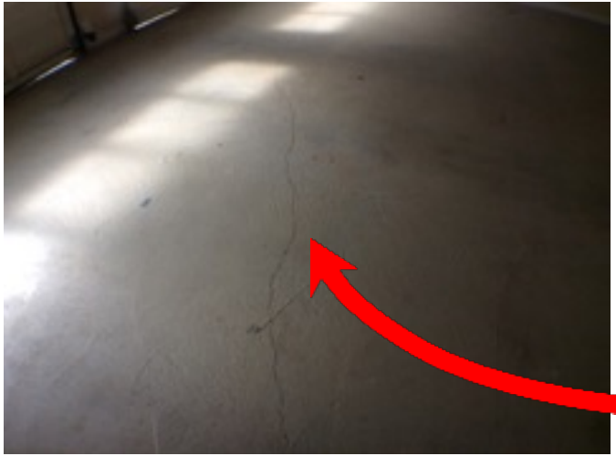
Garage Flooring Crack in flooring.
