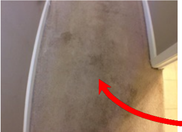
Flooring - Stains in Flooring.
