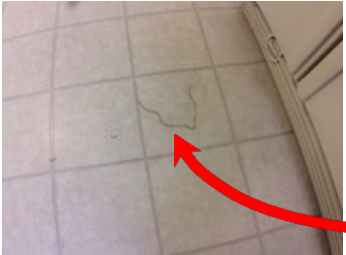
Kitchen Flooring Tear in floor.
