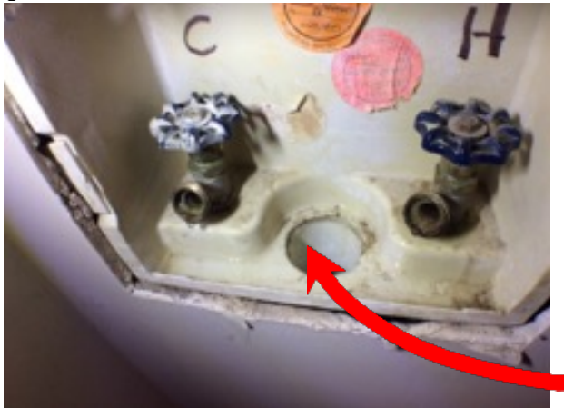
Washer Connection - Faucets were leaking.
