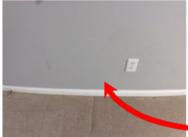
Walls/Paint - Marks on wall.
