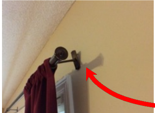
Blinds/Drapes - Curtain rod pulling away.
