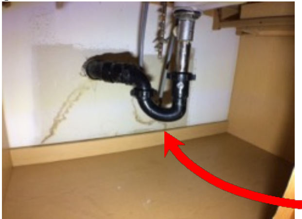
Cabinet Under Sink - Discolored rear of cabinet.
