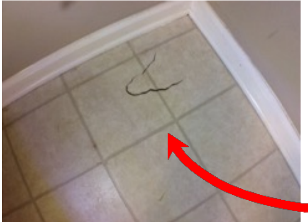
Flooring - Tear in floor.
