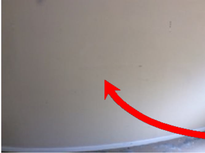
Garage Walls/Paint Marks on walls.
