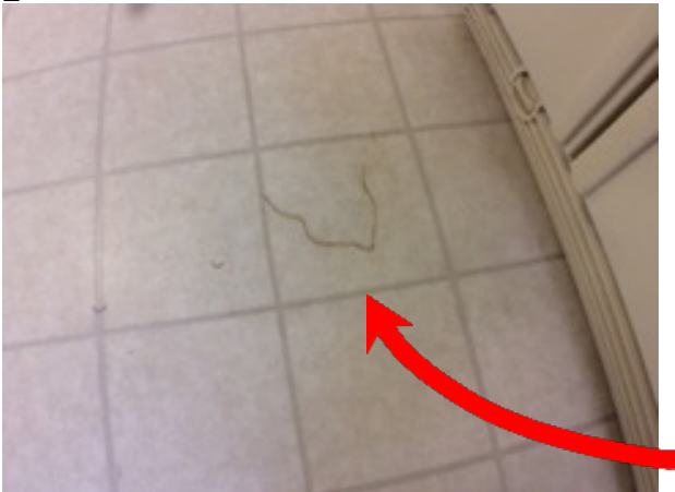
Flooring - Tear in floor.
