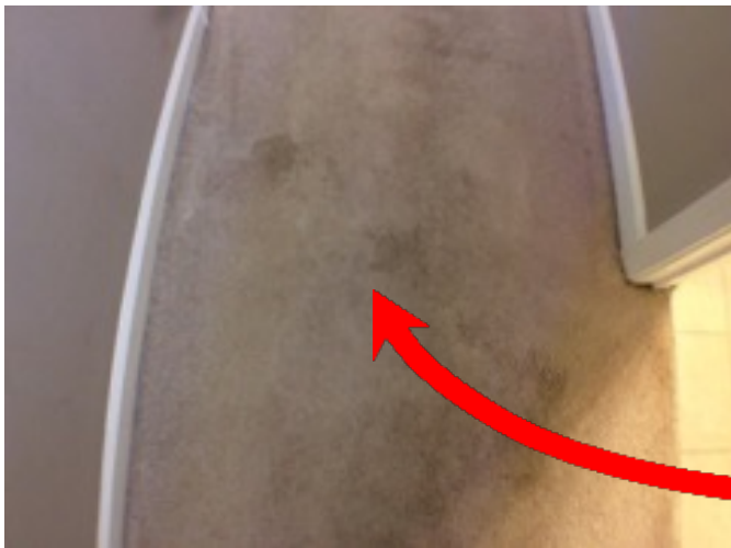
Hallway/Stairway Flooring Stains in Flooring.
