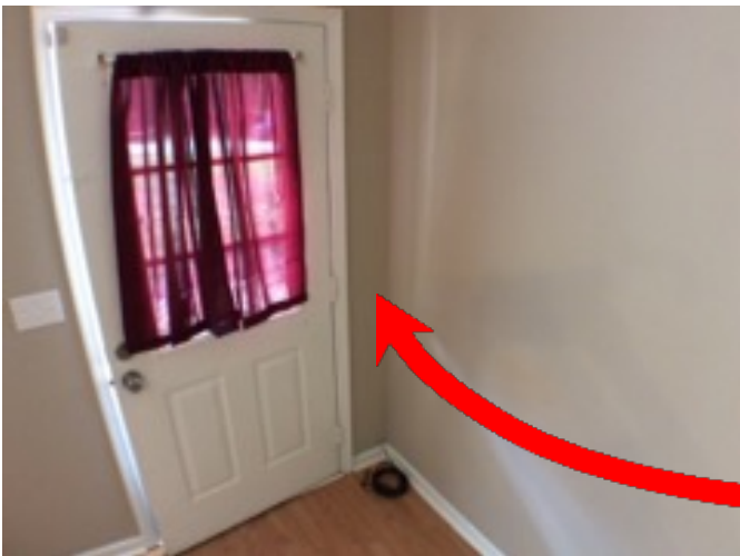
Entry Door Stops Missing- no wall damage noted.
